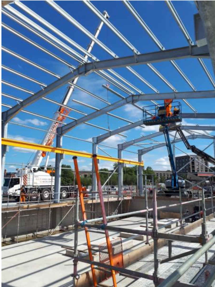
5 - Ibrox Pumping Station
