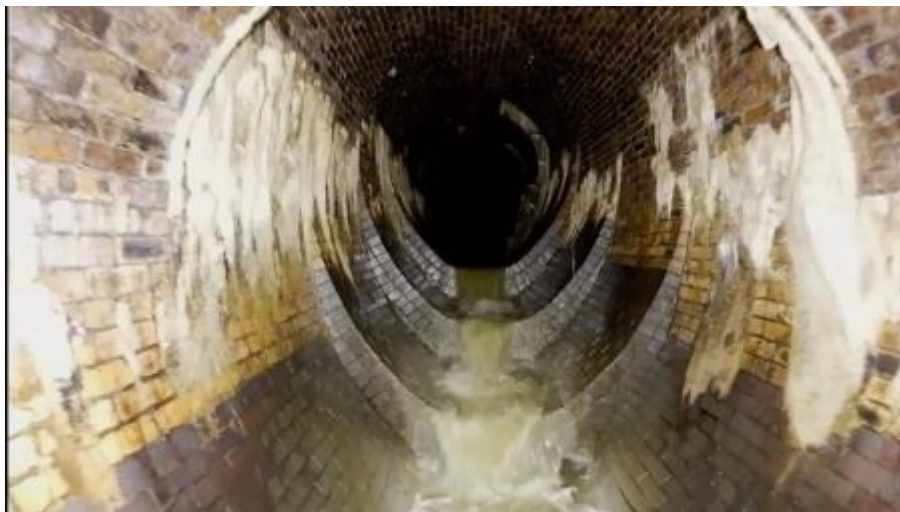
15 - Drone and AI technology is helping map our 33,000 mile sewer network - going where no man has gone since they were built by the Victorians. It also saves carbon emissions.
